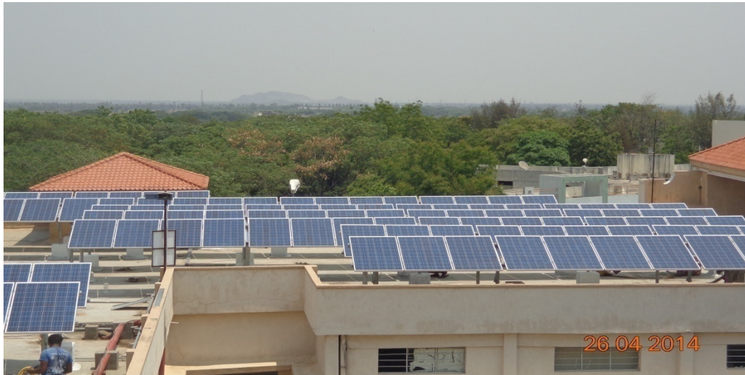
Fig- Roof Top Solar Energy Generation system
